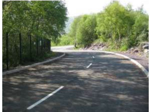
8. View south - Loosely surfaced footway at either side of newly constructed highway.
