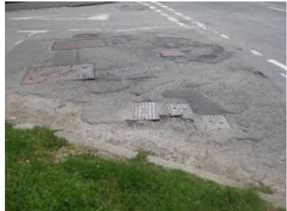
38. Existing service covers at western side of A4085 at its junction with unnamed road from Croesywaun to Groeslon, areas of degradation to the highway covering the width of the lane.
