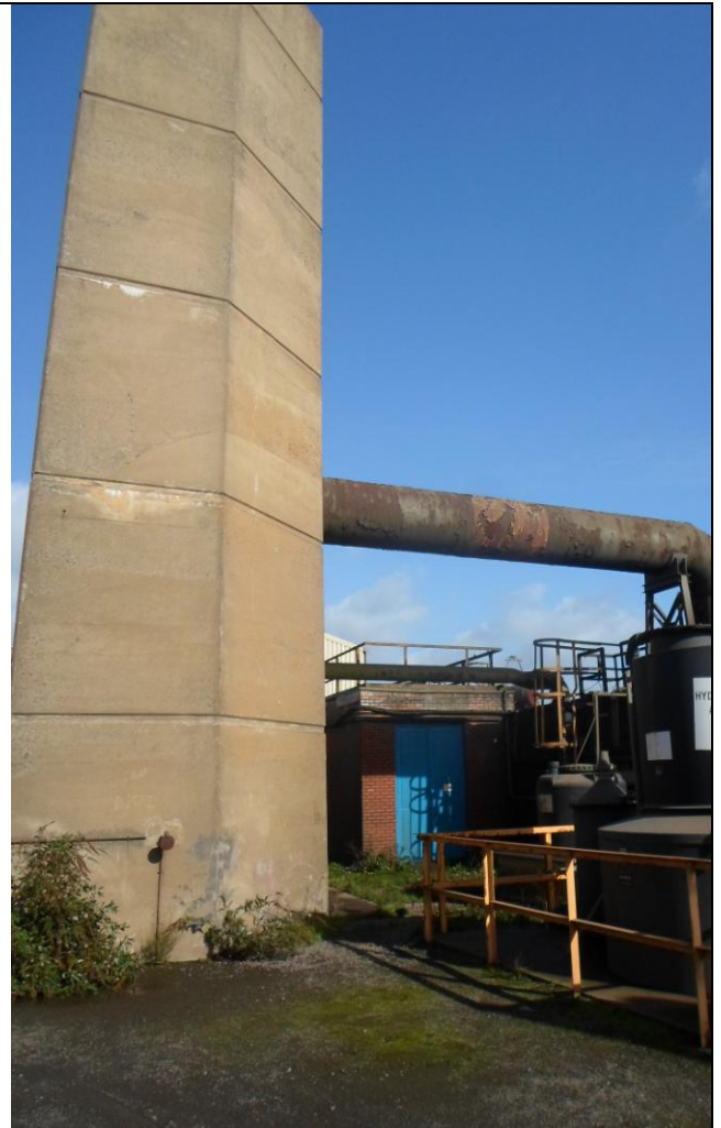
Photograph 10: Pipe work and pump house for Margam no.2 Sump. Discharge water is gravity fed to the long sea outfall.
