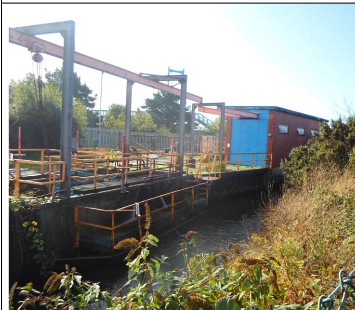
Photograph 7: Pump station and abstraction point from the Port Talbot Dock Feeder Channel sourced from the River Afan.
