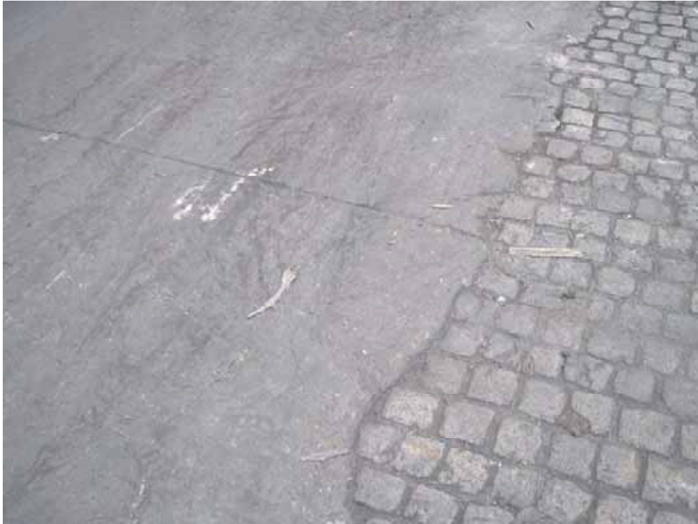
Pavement Surface – Henry Bath Shed
