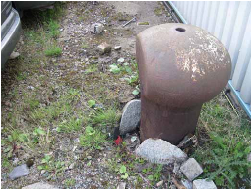
Disused Bollard & Damage Ground – AAA Car Auctions
