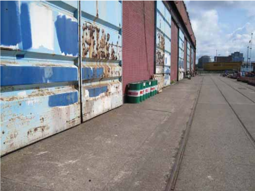
Empty Oil Drums – Alexandra East Shed
