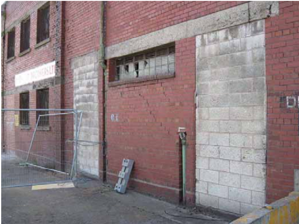
Cracking in Alexandra West Shed
