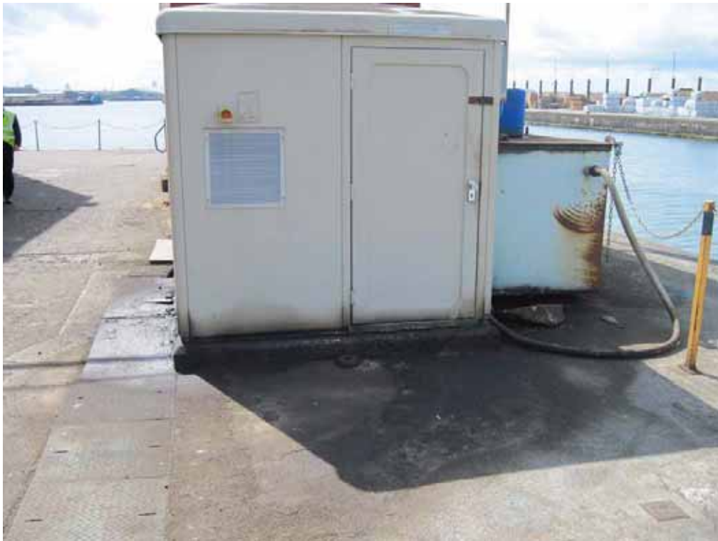
Canada 90' Swing Bridge Hydraulic Controls
