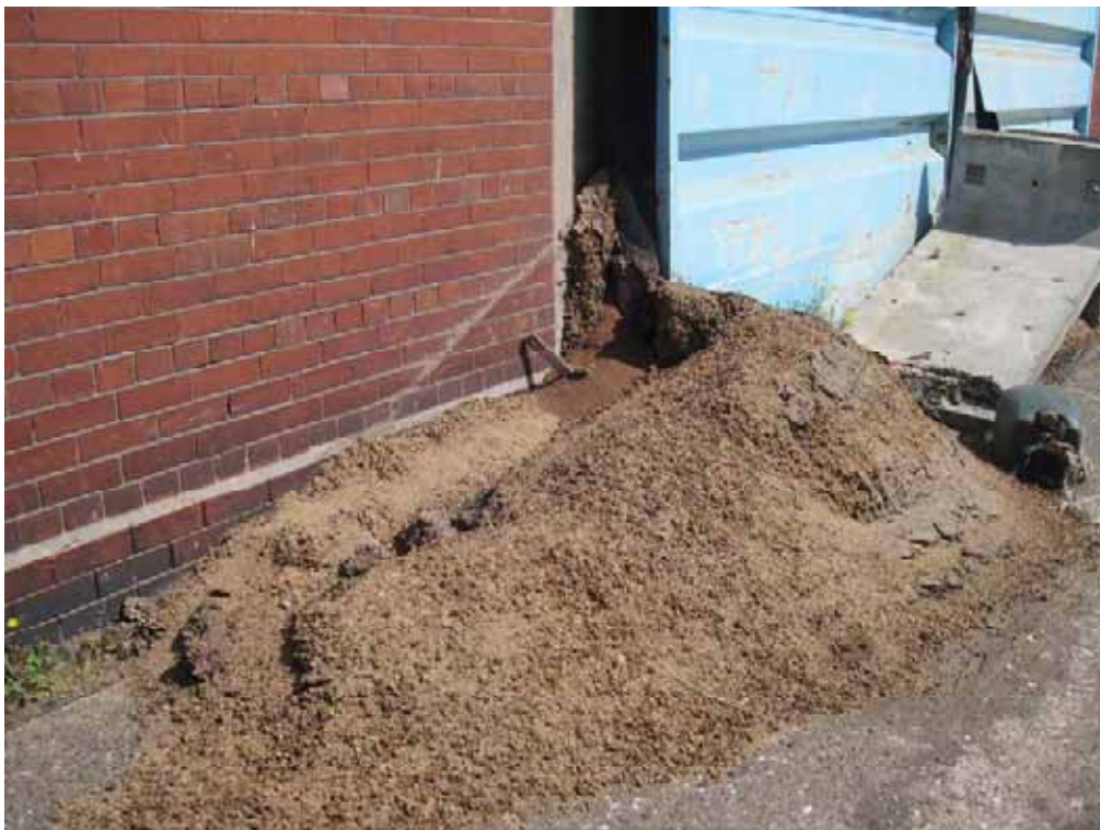
Grain Overflow Through Door – Alexandra Central Shed
