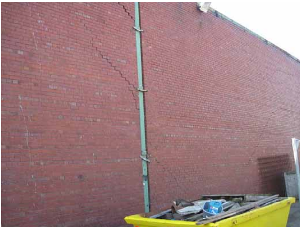
Cracking in Alexandra West Shed
