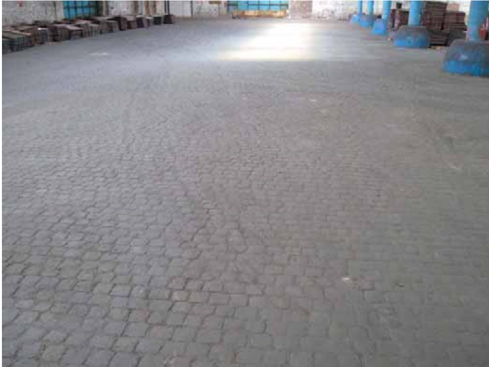
Pavement Surface – Henry Bath Shed
