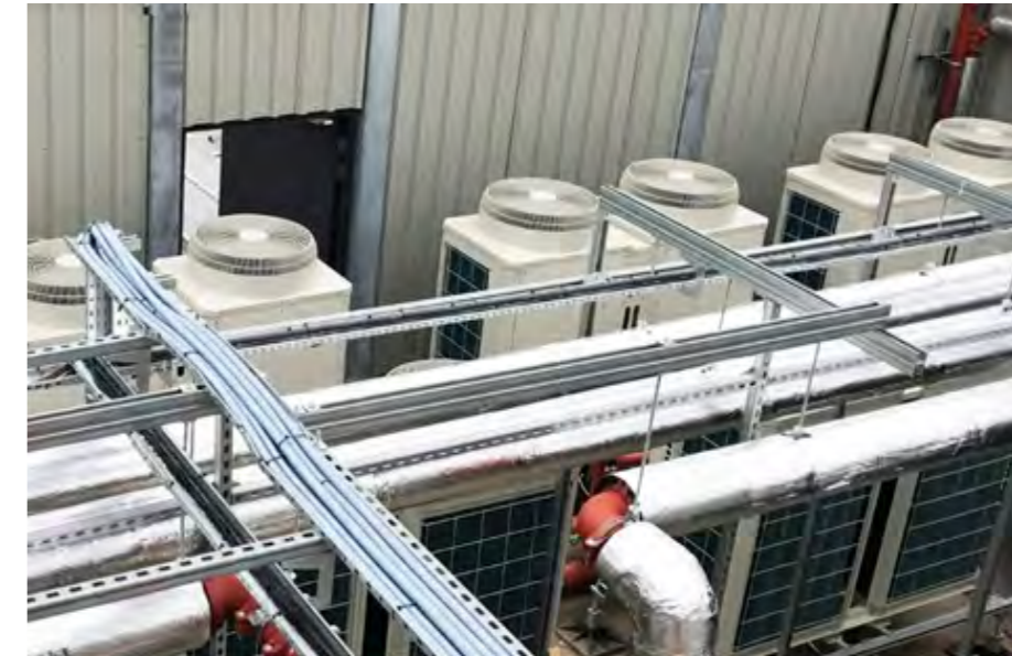
Figure A.56: Air Source Heat Pumps
