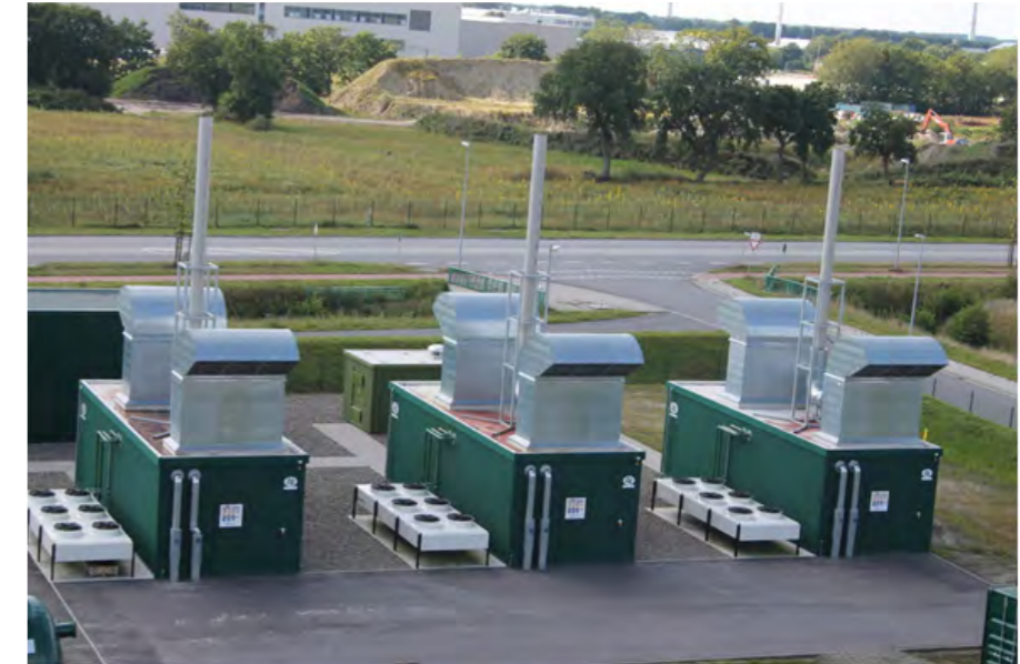
Figure A.55: CHP Generator
