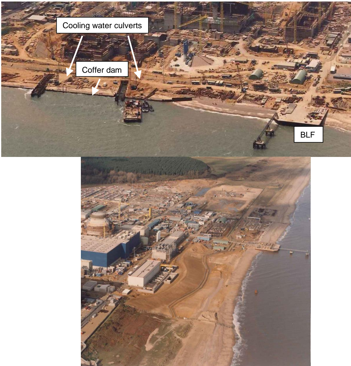
Figure 25: Aerial photographs of the coast during Sizewell B construction. Oblique aerial photograph looking west, showing details of the beach landing facility (BLF) on the right and the intake and outfall culverts on the left (May 1990). Note the removal of the beach and replacement with coffer dam at a position landward of the adjacent shoreline. The resulting bay is likely to be the result of dredging for the cooling water culverts. Bottom: North looking aerial photography (November 1992) following removal of the culvert coffer dam showing the partly constructed sea defences and the embayment formed at the position of the coffer dam and in the lee of the BLF.
