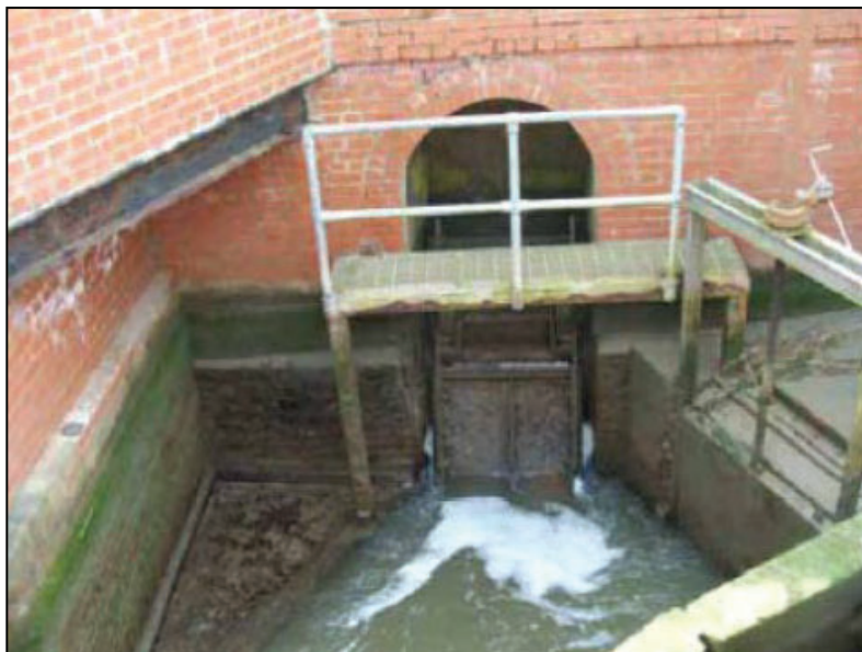
Plate 1.4: Leiston Drain flapped outfall, prior to remedial work (JBA, 2013).
