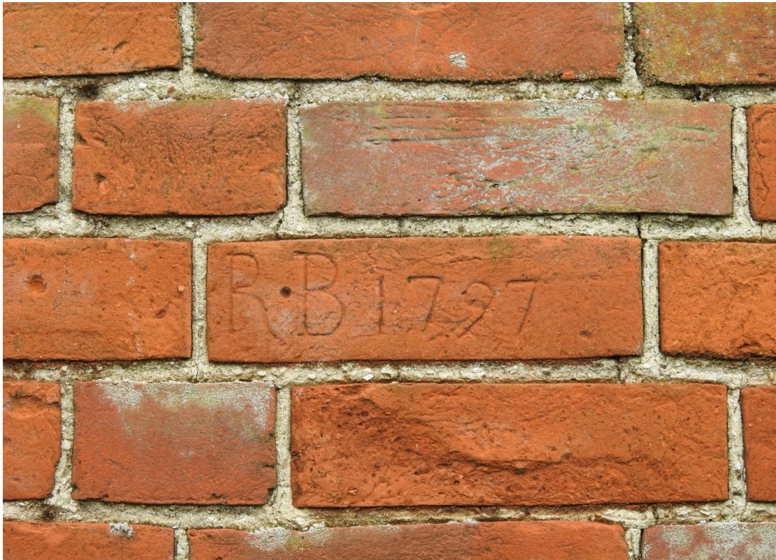
Illus. 20. A detail of the third of the three sets of initials neatly incised into the brickwork of the cart lodge's northern external gable (3), all dated 1797: From top to bottom 'Z K', 'M B' and 'R B' (the latter shown here). A fourth set, 'S P' is followed by what appears to be the number '3'. The style of lettering is convincing and the structure probably dates from this year. 'M B' and 'R B' may be Daniel Barker's antecedents.
