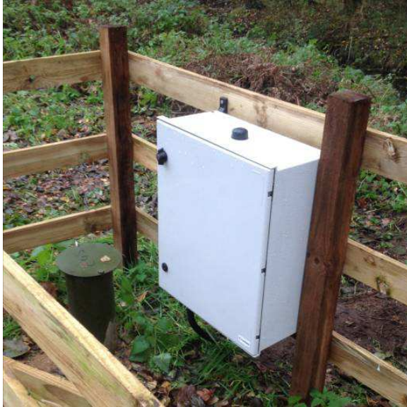
Figure 10: Photo of the enclosure (Site 6)
