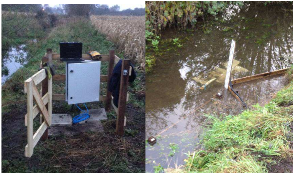
Figure 7: Photos of the installation at site 6
