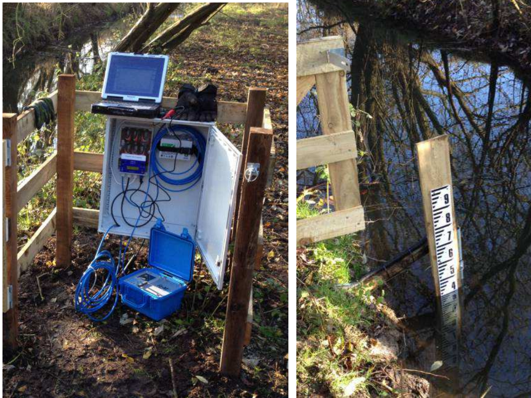
Figure 14: Photos of the installation at site 7
