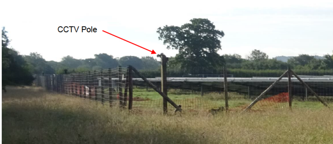
Insert 35: CCTV Pole and Fencing
