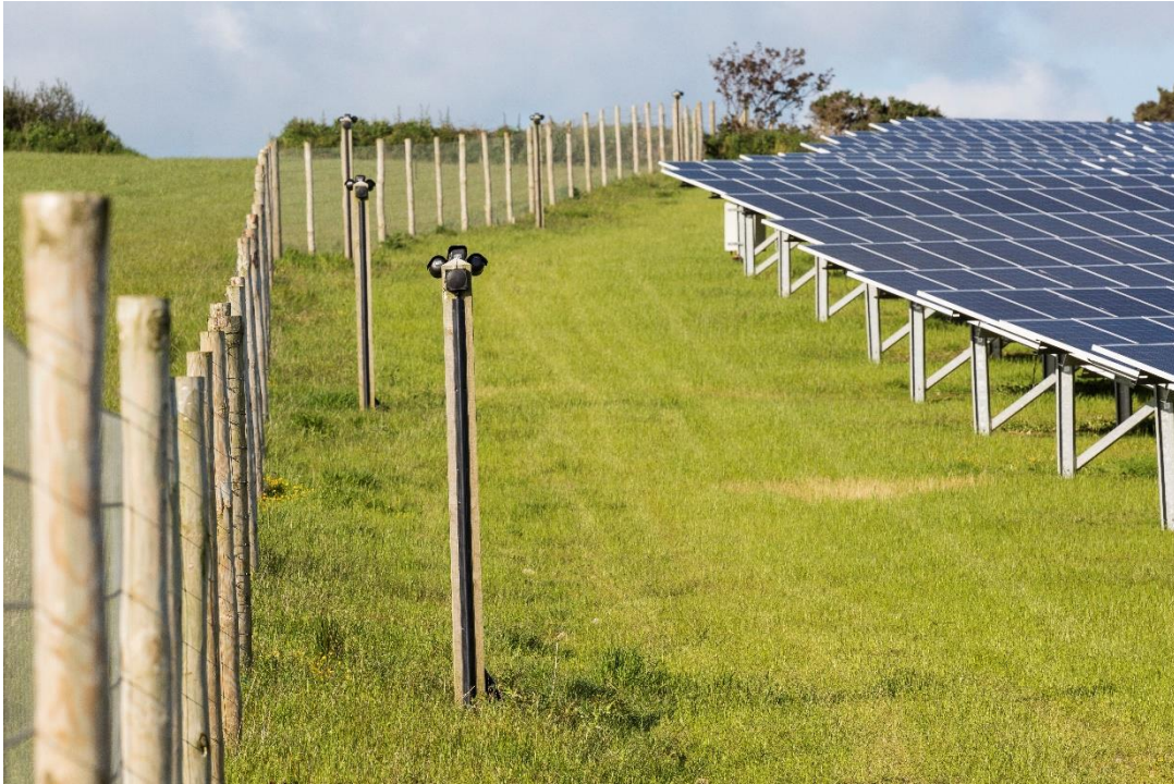
Plate 4: Example of security fencing and monitoring cameras
